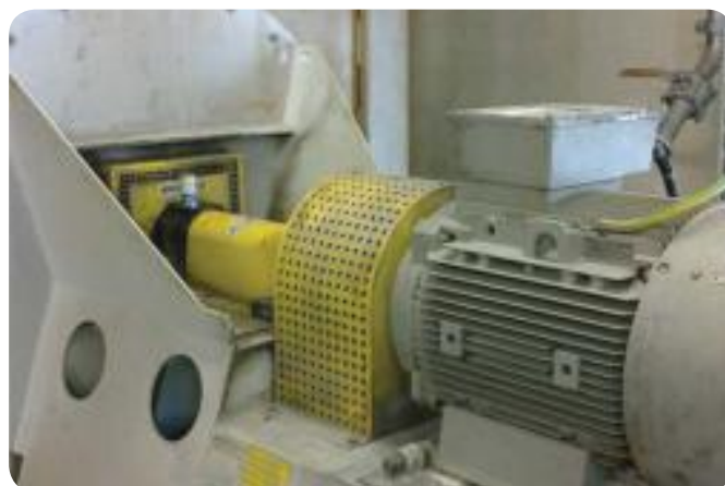
Fig. 1. Actual SKF Machine Condition Indicator installation.
